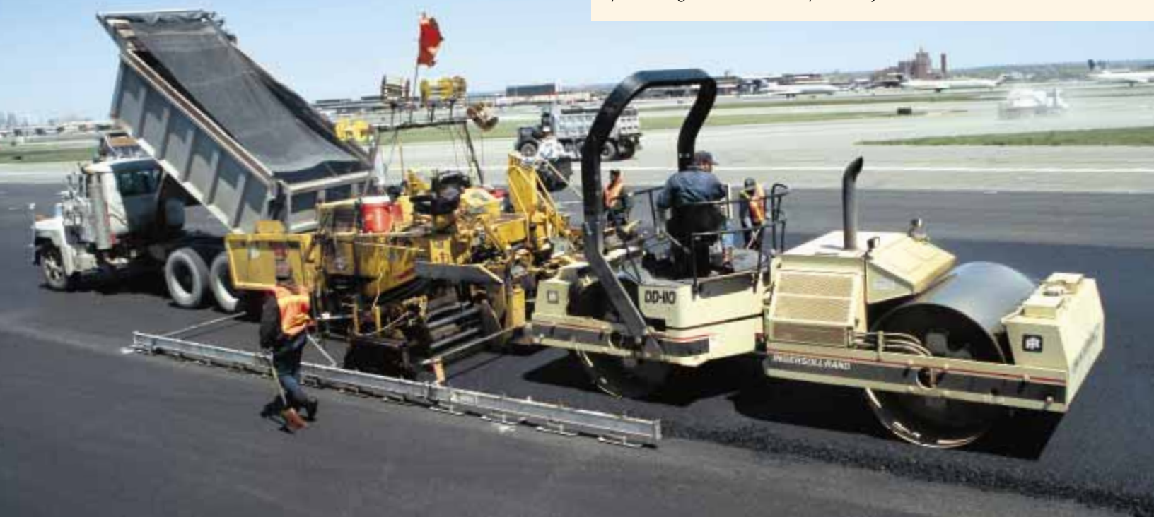
Working on a tight deadline, three Ingersoll-Rand compactors and two I-R Blaw-Knox asphalt pavers resurfaced one of the busiest runways at one of the busiest airports in the United States: Newark (New Jersey) International Airport. The units worked virtually nonstop for 15 days and nights, with nighttime illumination provided by 31 I-R portable light towers, to complete the job on time.
