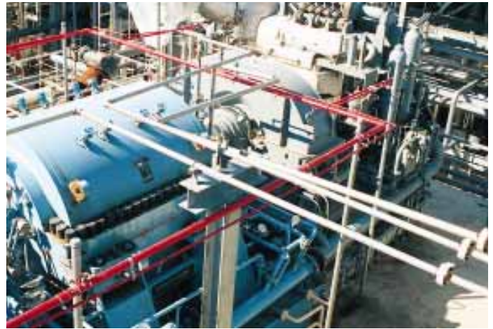
Dresser-Rand DATUM centrifugal compressors have demonstrated considerably greater ease of maintenance at Westlake Petrochemicals Corporation's ethylene plant in Sulphur, Louisiana
